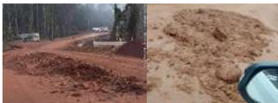
Figure 1. Limonite spill on Hauling Road
